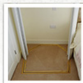
View of upstairs looking at the safety lid plug.
